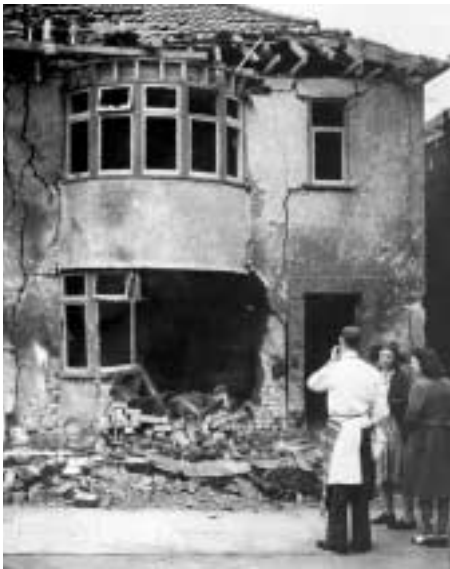
Damaged Bristol house
